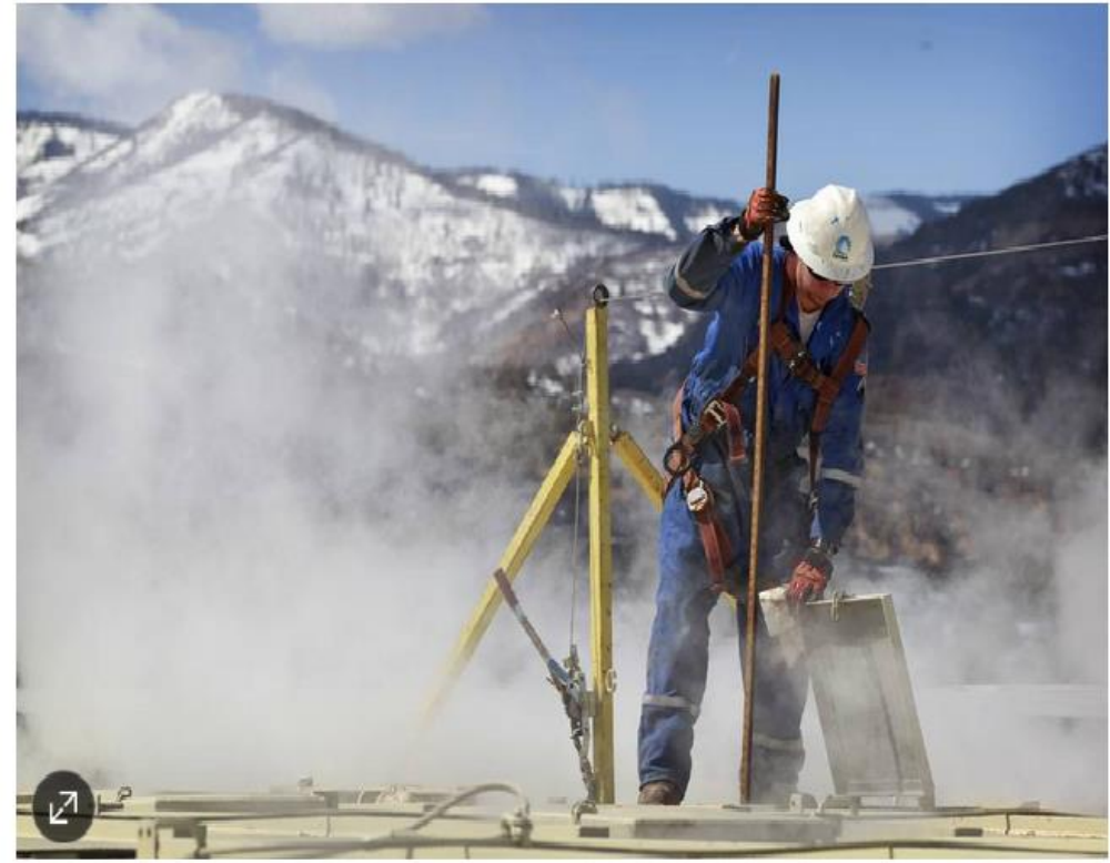
A worker checks water levels and temperatures at an Encana Oil & Gas hydraulic fracturing operation outside Rifle, Colo. PHOTO: BRENNAN LINSLEY/ASSOCIATED PRESS
