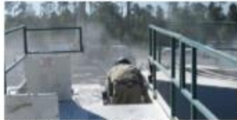
Silica dust cloud by worker delivering sand from sand mover to transfer belt.
